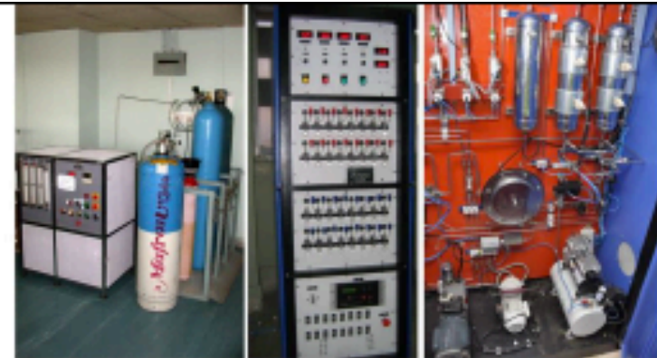
Closed loop gas system
