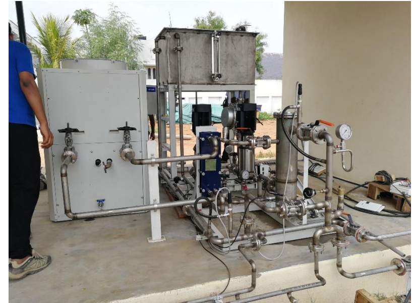
Low conductivity water cooling system for magnet & power supply
