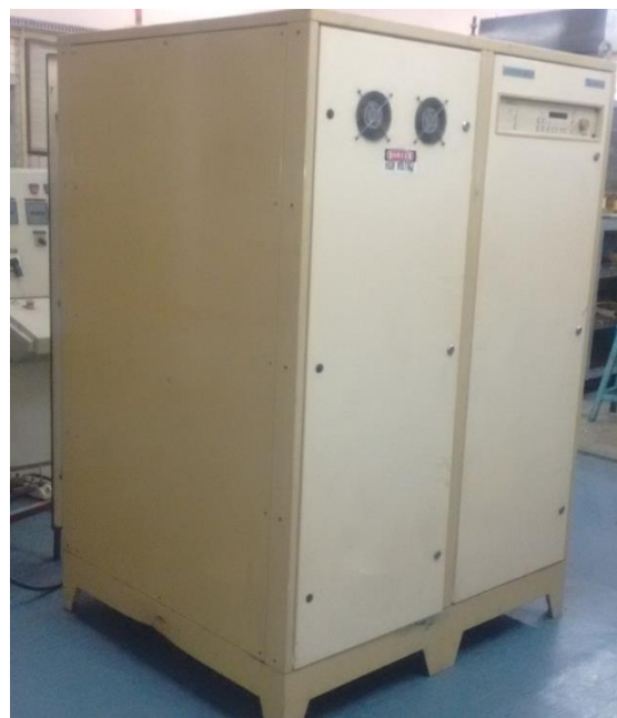
Magnet power supply 30V DC, 1200 AMP
